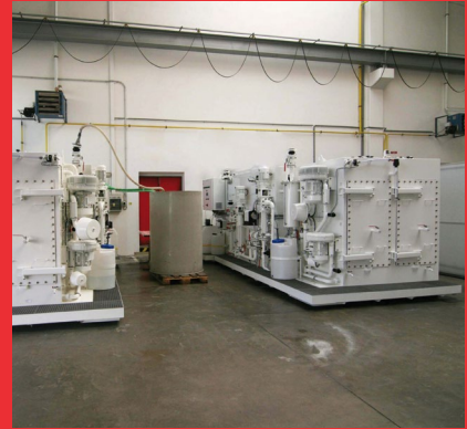
Sewage Treatment Systems
